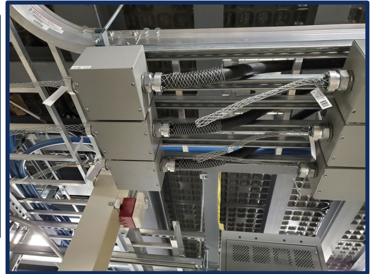
Pre-located J-boxes for HPC Rack Power Whips
