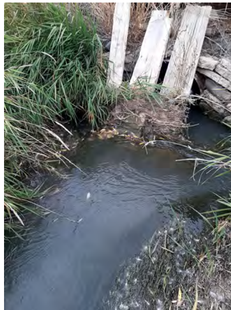
Figure 5. Boards placed in front of culvert to prevent blockage of the structure.
